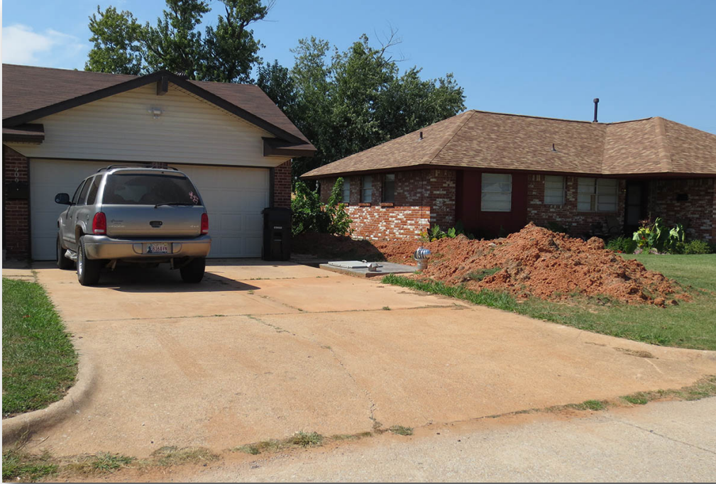
Fresh piles of dirt can be seen in many front yards where underground storm shelters have recently been installed. The two homes pictured are older homes about a block north of the Plaza Elementary, and were spared from the tornado.
